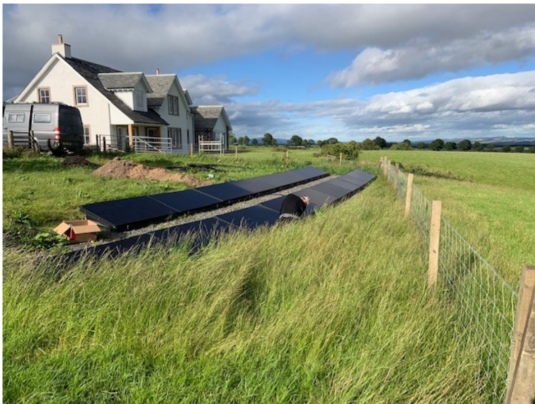
Figure 9 – Example image of ground mounted solar panels
