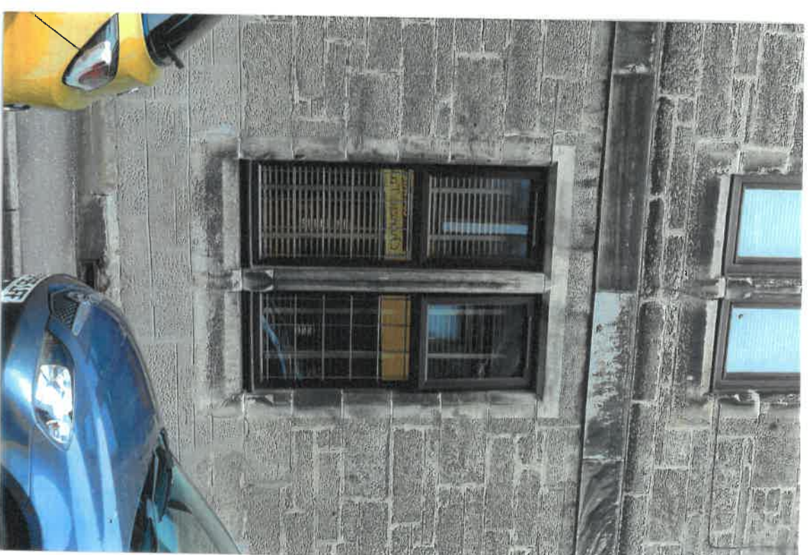
PHOTO OF EXISTING FRONT ELEVATION WINDOWS ADJACENT TO RIGHT SIDE OF ENTRANCE DOOR NO 163, MAIN ST. LOCHGELLY.
