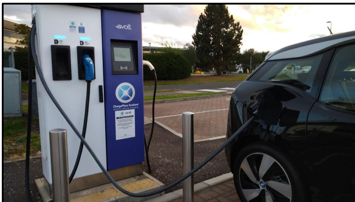
Figure 2-8 Rapid charger in Fife
