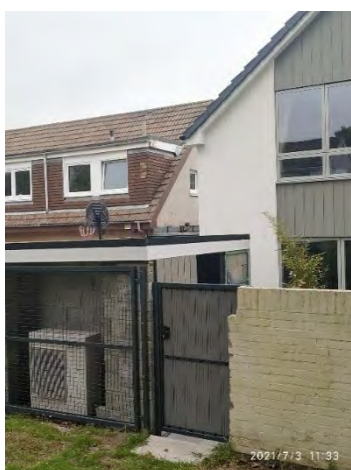
Photo 14: This is a plantroom, not a shed.
