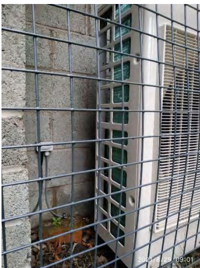
Photo 13: Coils and other electric parts of the outer unit
