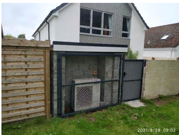
Photo 2: The ASHP and its plantroom
