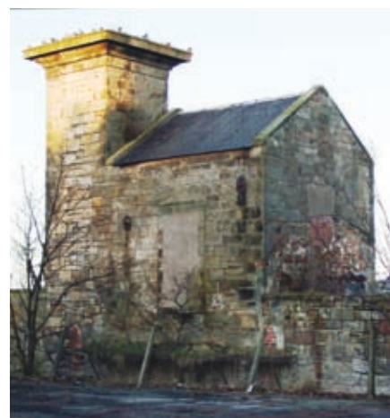
The former Sawmill chimney building is a local landmark whose preservation could form the focus of a redevelopment proposal
