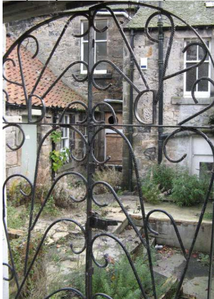
View of the back of the Dundonald Arms. Broken window panes, failing rainwater goods and growth of vegetation indicate decay as a result of being unoccupied.
