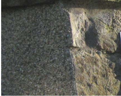
Example of dry dash applied to one face of rubble wall, likely to disrupt the normal processes of moisture movement through the wall
