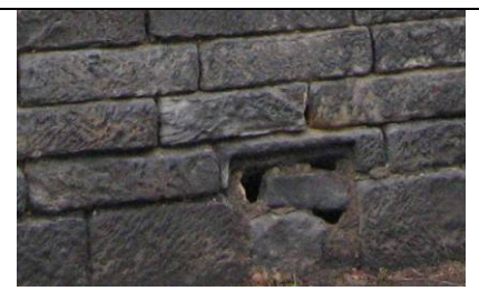
Missing ventilation grille
