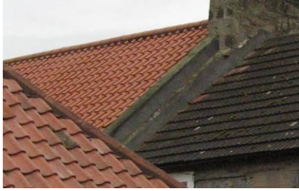
Roofscape at West Green: left, historic clay pantile, middle, modern pantiles, right, concrete roof tiles.
