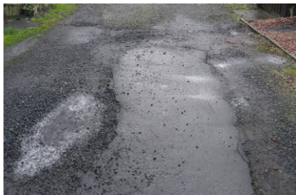
Asphalt in poor condition on Back Street
