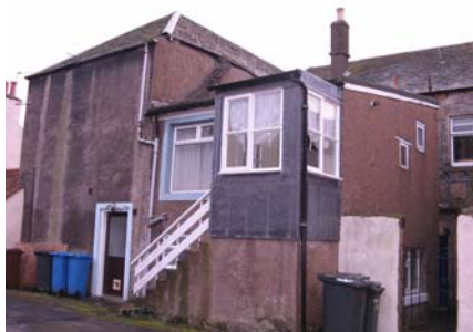
These 20 th century additions seem haphazard and detract from the streetscape.
