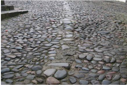
A sunken section of causeway paving is to be seen at the top of Mid Causeway near the Mercat Cross.
