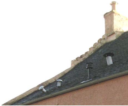
Protrusions on the roof of a front elevation, Low Causeway
