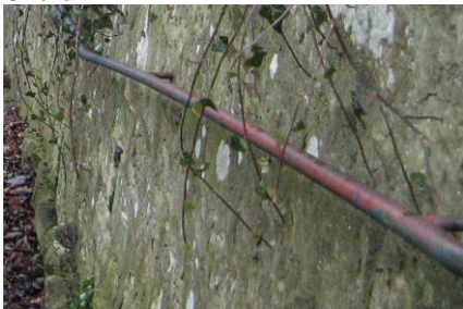
The handrail on Hagg's Steps needs maintenance or renewal.
